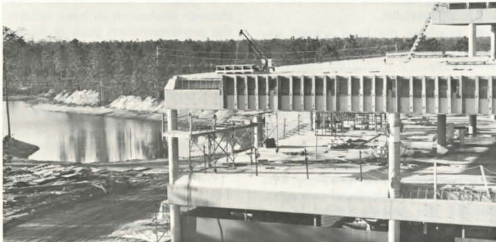
The University of North Florida building complex is progressing faster than expected. Wesley of Florida is ahead of their construction schedule which will put the UNF administration and staff into the administration and library buildings by July. The classroom and laboratory buildings will be ready for occupancy by Sept.
