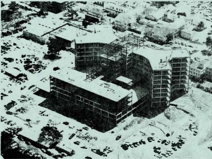
This bird's eye view of the new medical center under construction gives a panoramic perspective of the hospital's design and layout. The eight-story double "Y" inpatient tower is separate from but co-ordinated with the five-story outpatient clinics (foreground). The power plant and laundry are in upper left with the present hospital in the background.
