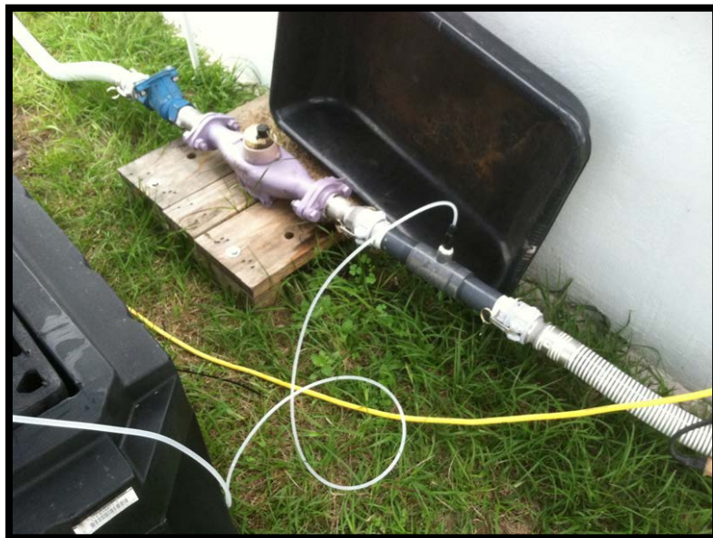
Figure 33 - PAA Injection Point with Inline Flowmeter
