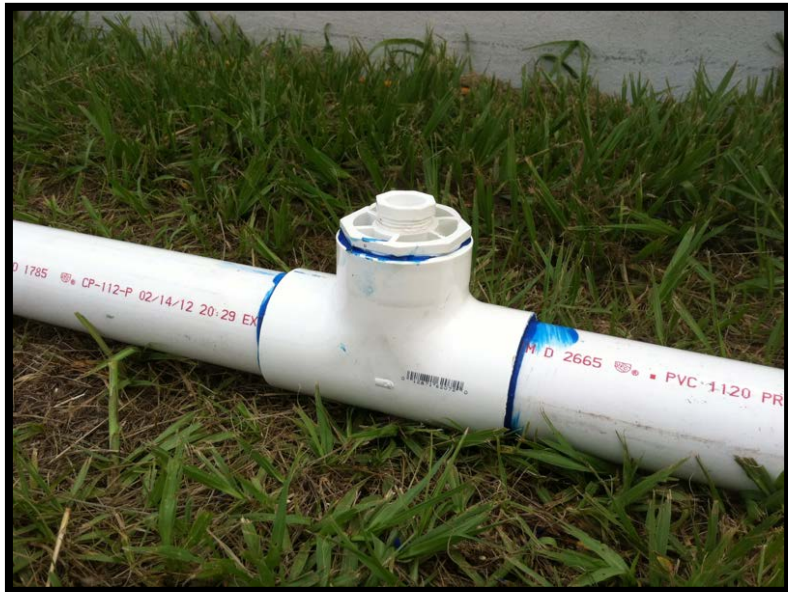
Figure 41 - PAA Injection Point
