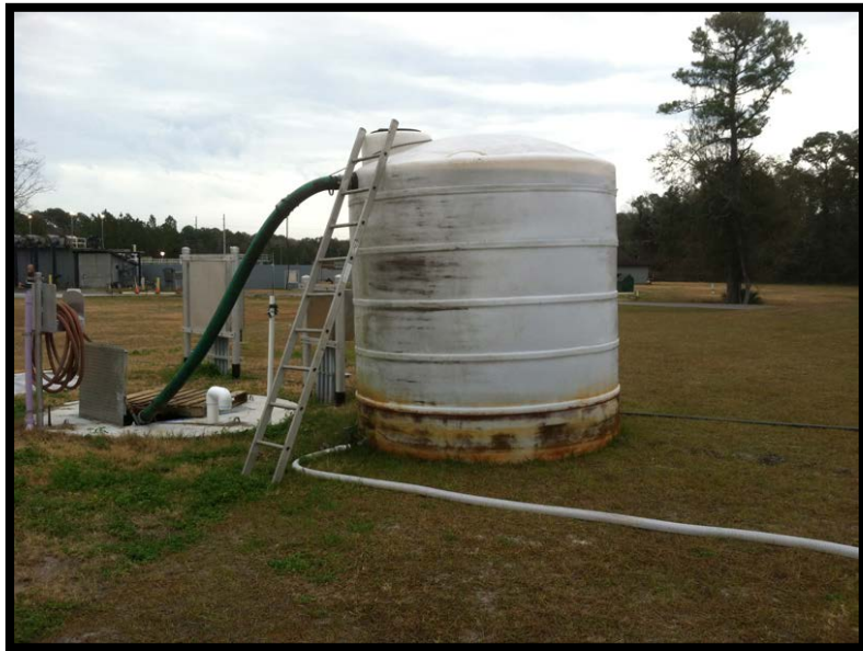
Figure 35 - Portable Tank Used for PAA Contact Chamber Discharging to Lift Station
