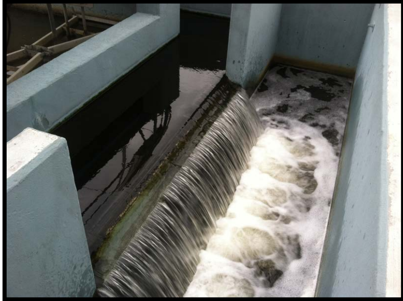
Figure 34 - Effluent Reservoir of Sand Filter
