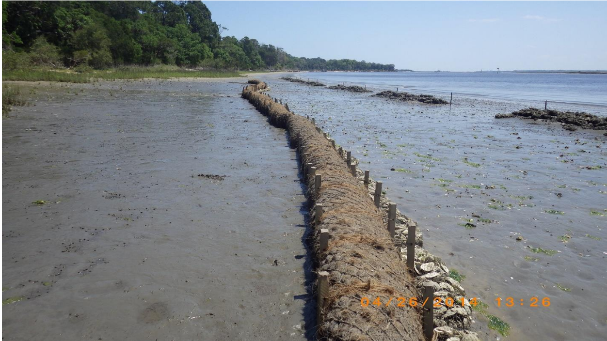
Figure 2-2 Deployed fiber (coir) logs along Wright's Landing in the northern Guana Tolomato Matanzas National Estuarine Research Reserve (30.0225250°N, 81.3262806°W) Florida, U.S.A. These logs were installed approximately 5-m from the existing Spartina marsh edge in the high intertidal zone. Logs were placed in 20-m arcs both behind constructed oyster reefs (pictured), and alone, along eroding shoreline.
