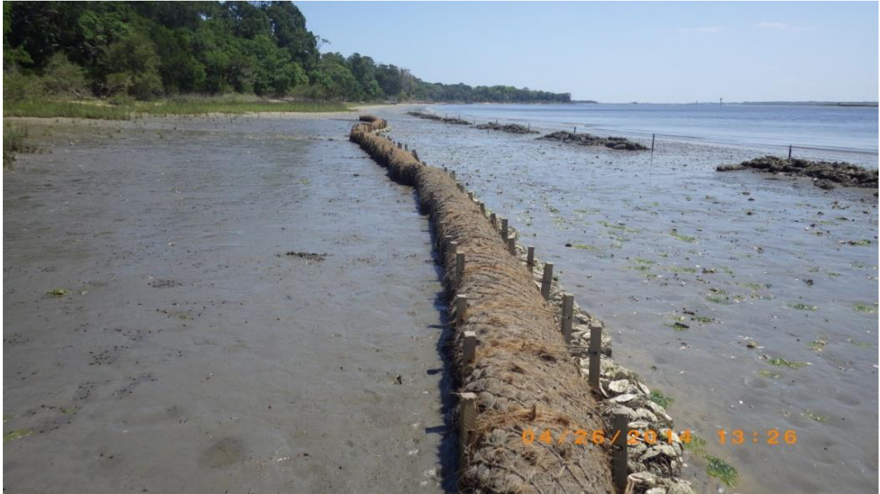
Figure I-3 Complete fiber log installation on the southern end of the existing artificial oyster reef along Wright's Landing in the northern Guana Tolomato Matanzas National Estuarine Research Reserve. Photo was taken April 26, 2014 following the installation. Logs were placed in 20-m arcs behind the constructed oyster reefs using wooden stakes and twine. Plastic mesh bags filled with oyster cultch were placed in front of the logs for stabilization.
