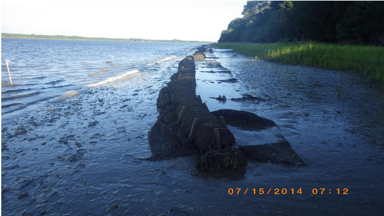
Figure I-4 Complete fiber log installation 100-m north of the existing artificial oyster reef along Wright's Landing in the northern Guana Tolomato Matanzas National Estuarine Research Reserve. Photo was taken July 15, 2014 following the installation. Logs were placed in 20-m arcs approximately five meters in front of Spartina marsh grass on unstructured eroding shoreline using wooden stakes and twine. Plastic mesh bags filled with oyster cultch were placed in front of the logs for stabilization.
